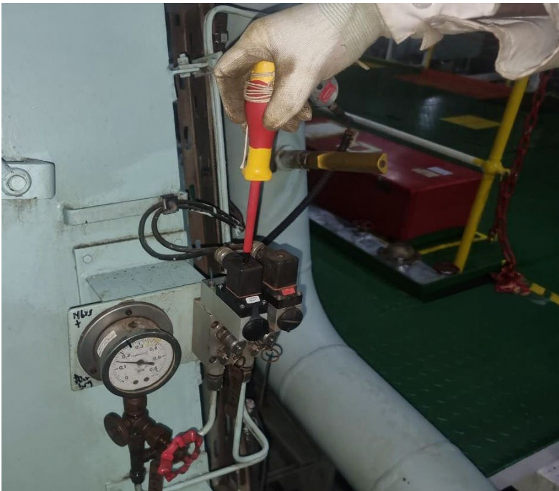
Figure 4: Main engine lubricating oil pressure sensing and switches
