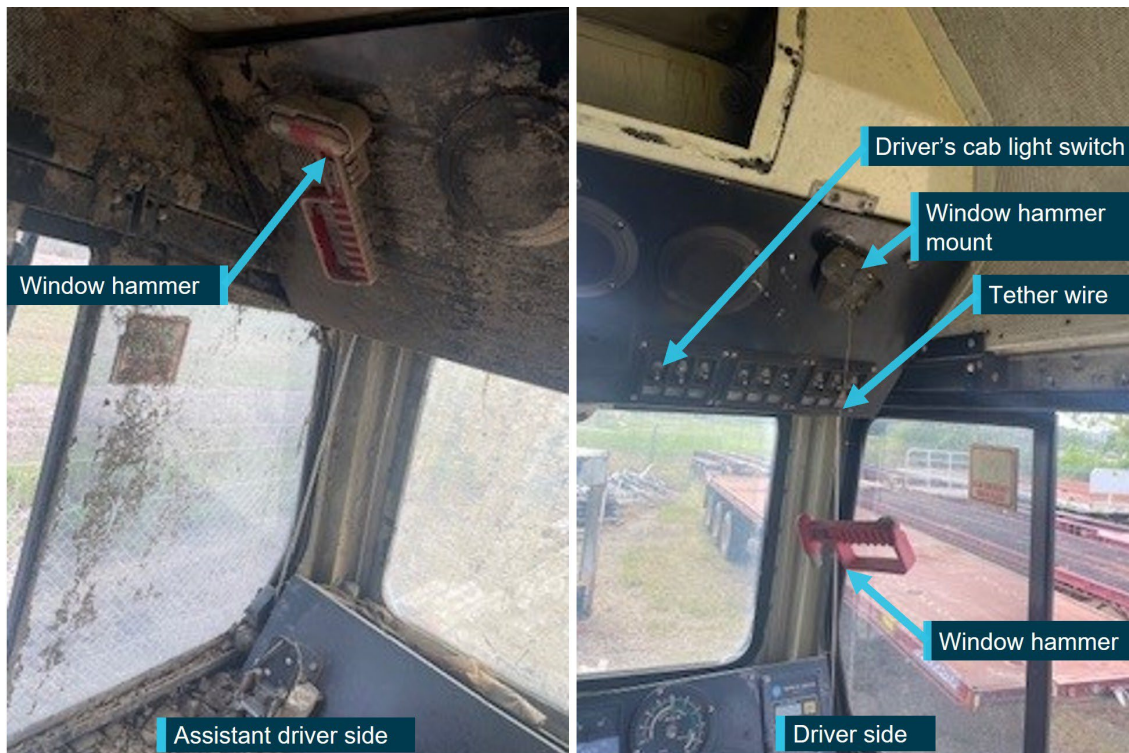
Figure 18: Window-breaking hammer installation in locomotive 2811 no 2 end cab
