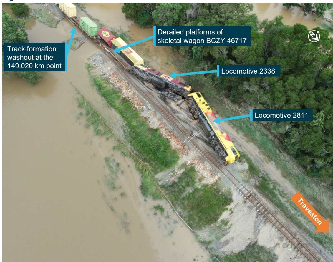
The image (taken later on the day of the derailment) shows derailed rail vehicles from train Y279, washout and other damage to the track formation. Source: ATSB
