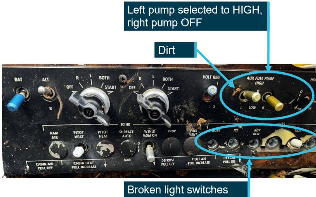
Figure 9: Panel showing post-impact switch positions and disruption
