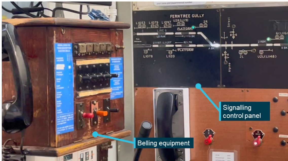
Figure 12: UFG belling equipment
