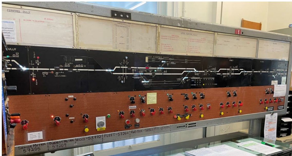
Figure 8: UFG station signal control panel
