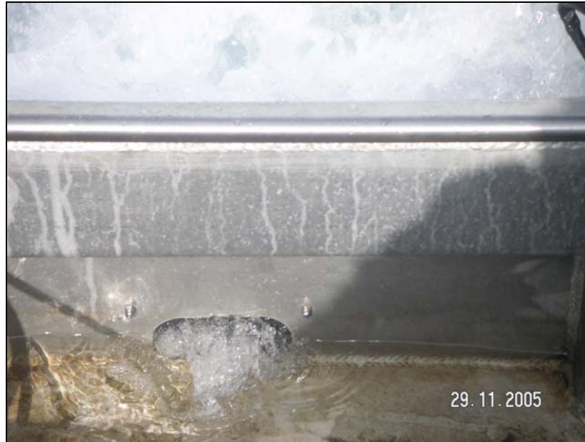
Figure 6: Water draining from the motor well
