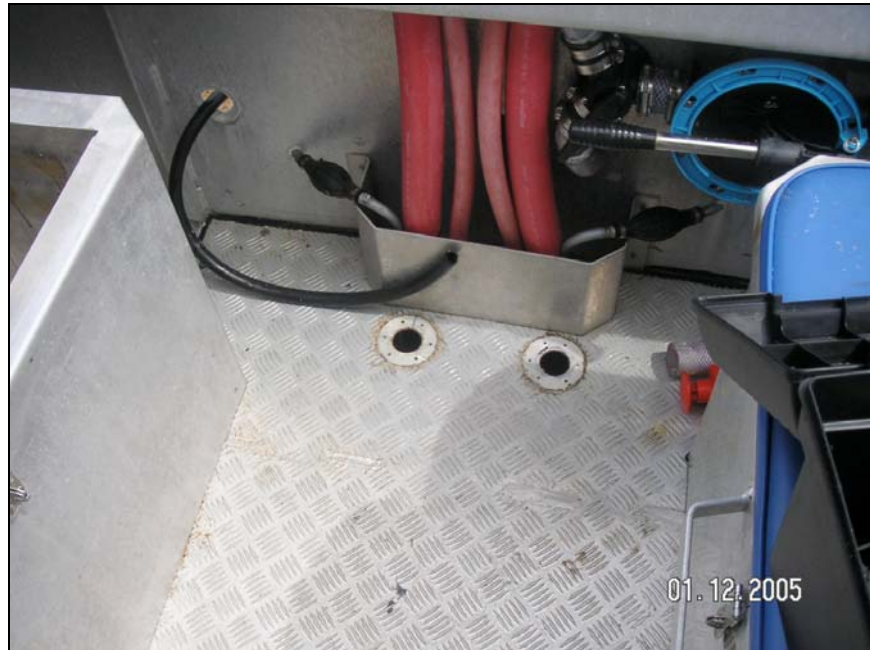
Figure 14: Top of fuel tank with hoses leading from up-stands
