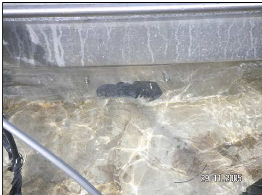
Figure 5: Water in the motor well
