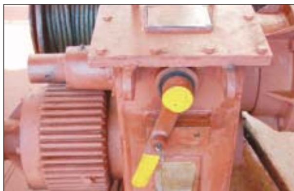
FIGURE 5: Clutch lever for hoisting winch for port lifeboat
