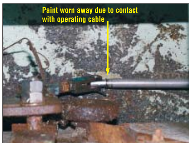
FIGURE 10: After hook operating cable system
