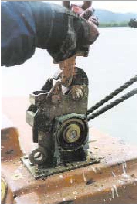
FIGURE 3. Lifting hook, plate removed
