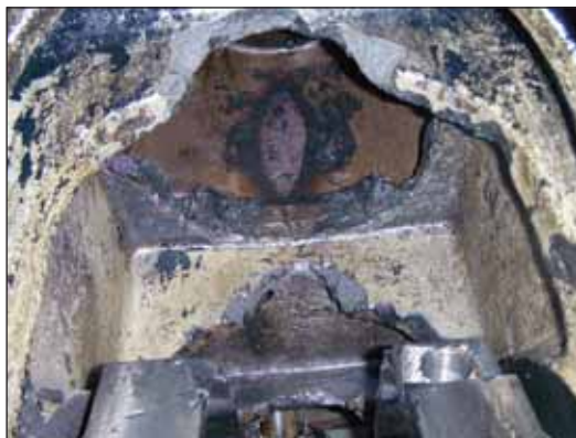
FIGURE 3: No.1 unit PME water jacket space
