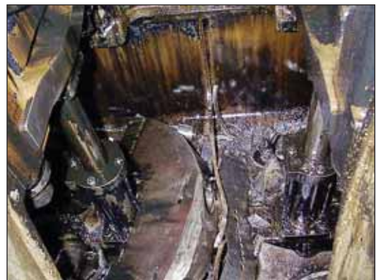
FIGURE 4: Debris in crankcase
