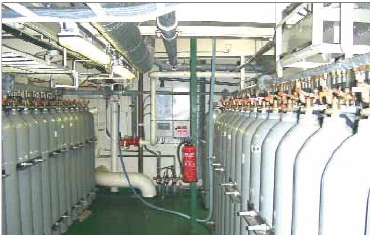
FIGURE 2: CO 2 room, showing banks of gas bottles for CO 2 flooding of cargo holds
