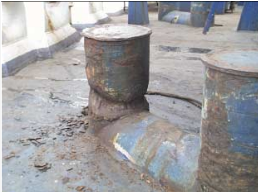
FIGURE 7 Damage to Ariake's mooring bits
